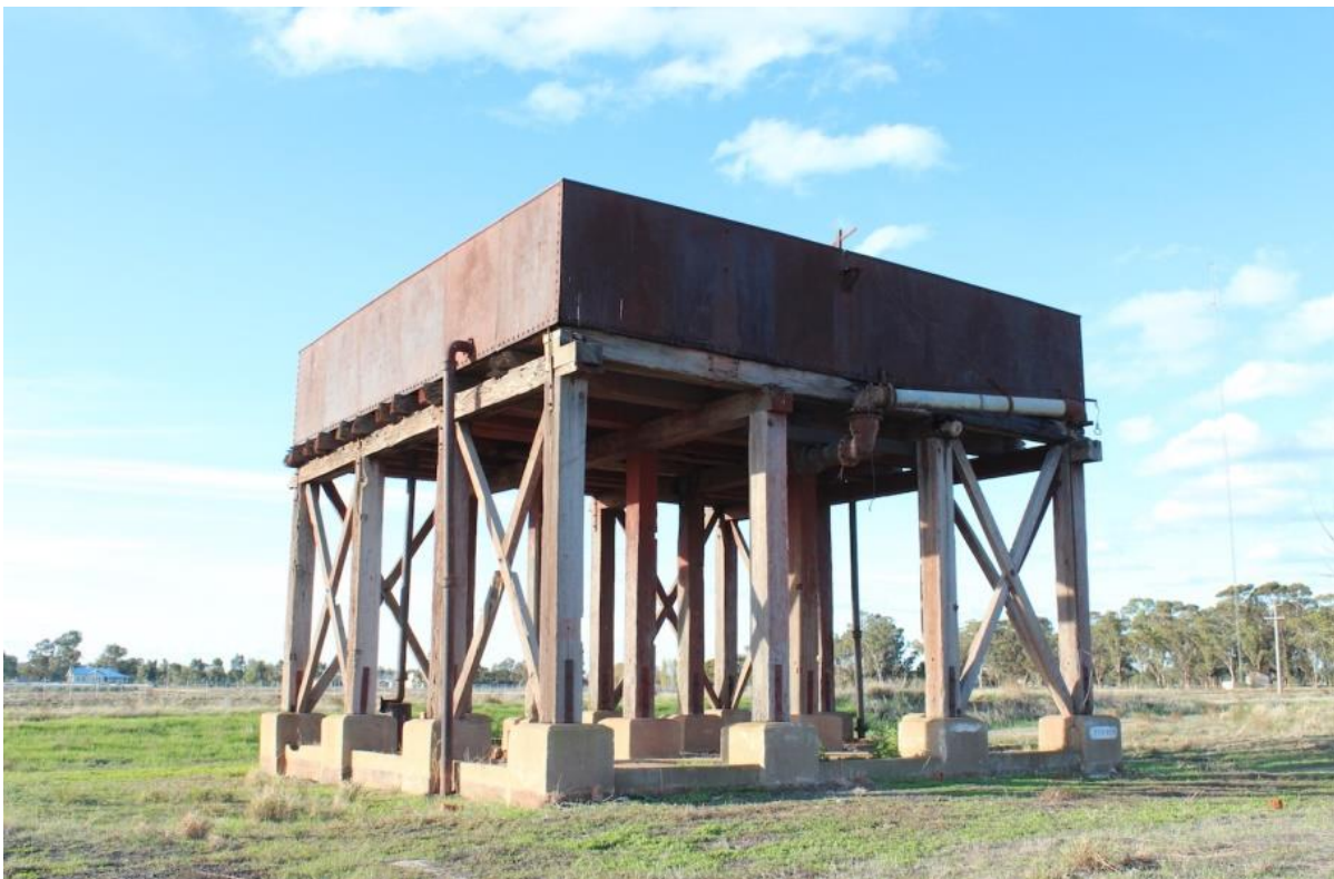
Figure 32. Early style of metal-plate water tank used on the NSW Railways (Source: Extent Heritage).
