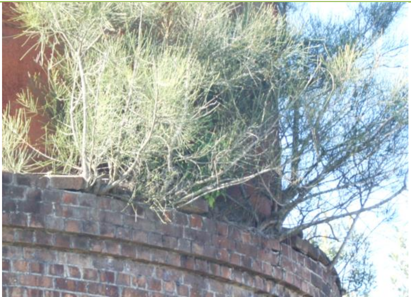
Figure 44. Brickwork around the upper rim is badly affected by vegetation growth.
