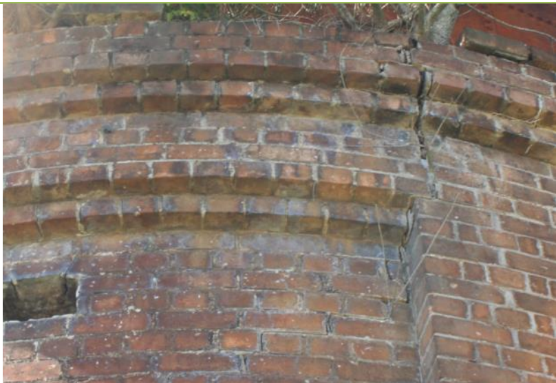
Figure 51. This brickwork crack is moving vertically downwards and is apparent on the inside of the brickwork as well.
