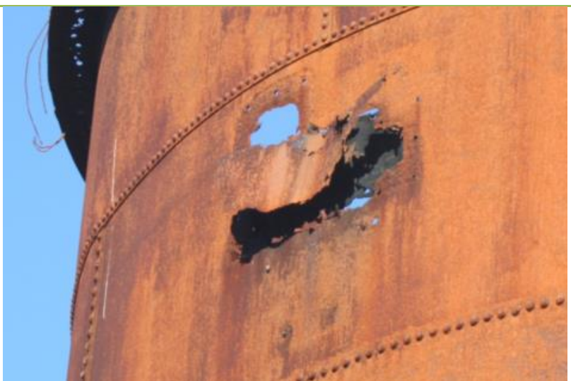
Figure 45. The metal work of the tank already shows evidence of previous corrosion repairs
