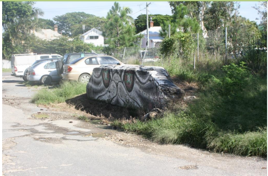
Figure 54. The southern concrete pier has been left standing, with the soil excavated from its southern side to form the present side road. It has been colourfully painted.
