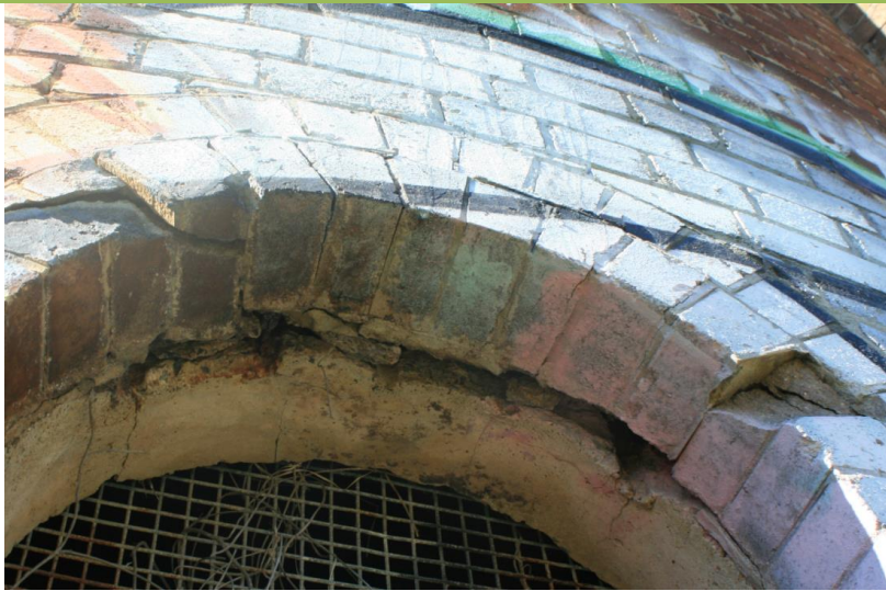
Figure 50. The arch brickwork of the western window has moved and one brick has been crushed.
