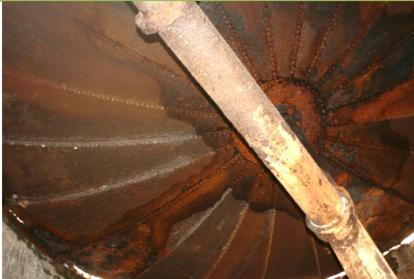
Figure 43. The underside of the water tank and outlet piping viewed from within the brick tower. The tank floor appears to be relatively sound.
