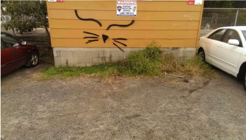
Photograph 14 The east elevation of the shed which requires protection A strategy for combating graffiti is recommended including artwork and interpretation.
