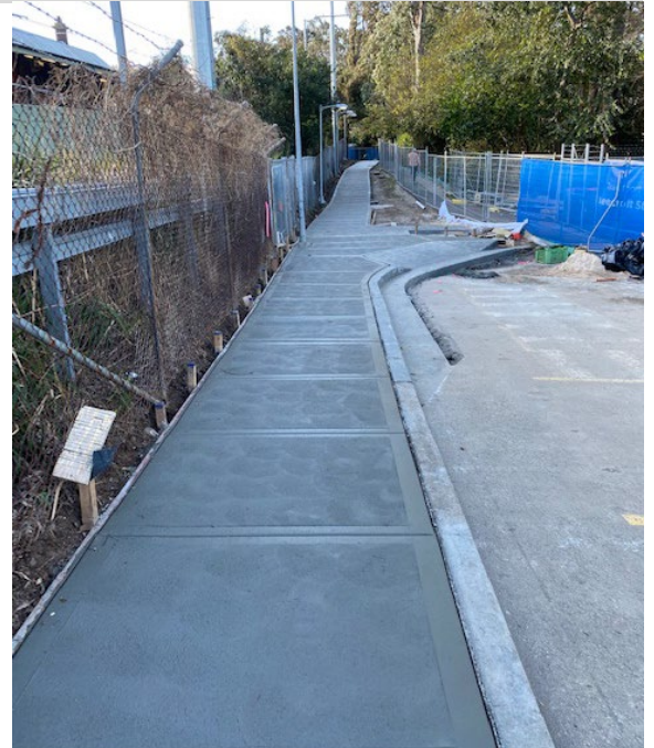
Pictured: Upgraded footpath between underpass and Sutherland Road Commuter Car Park. Late July 2021
