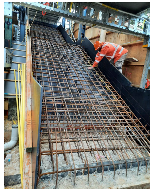
Image: Stair construction inside the platform hoarding. Detail measurements being taken by Site Engineer, Jan 2021
