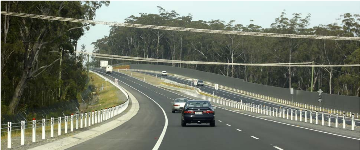
Smooth topped, plain concrete noise walls painted in a recessive colour, with vegetation to the rear and front.
