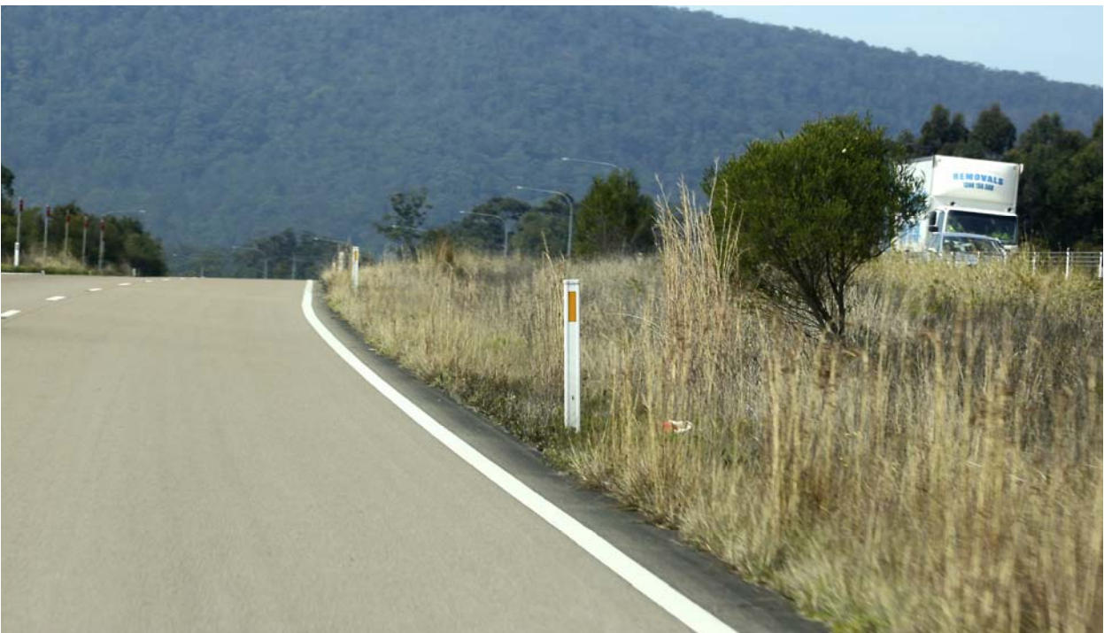
Independently graded carriageway on Karuah Bypass. This approach creates a more interesting fitting alignment.
