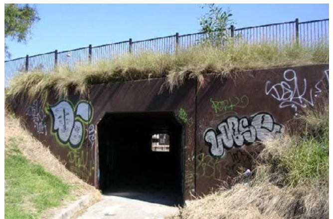
Graffiti litter and poorly maintained verges do not help what is already a very substandard underpass.
