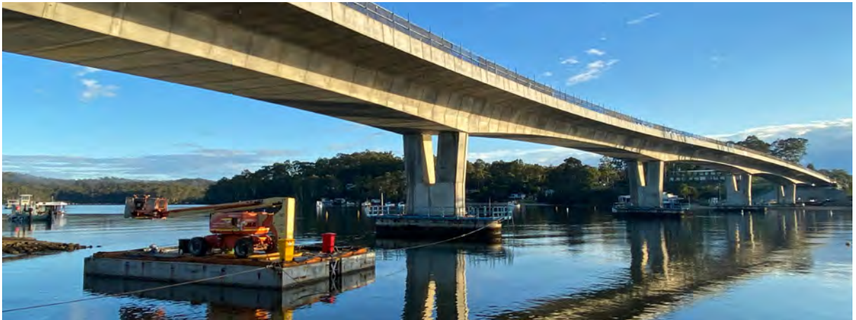
A beautiful bridge in the making, a river and a town renowned for its fishing and seafood. Quintessential South Coast.
