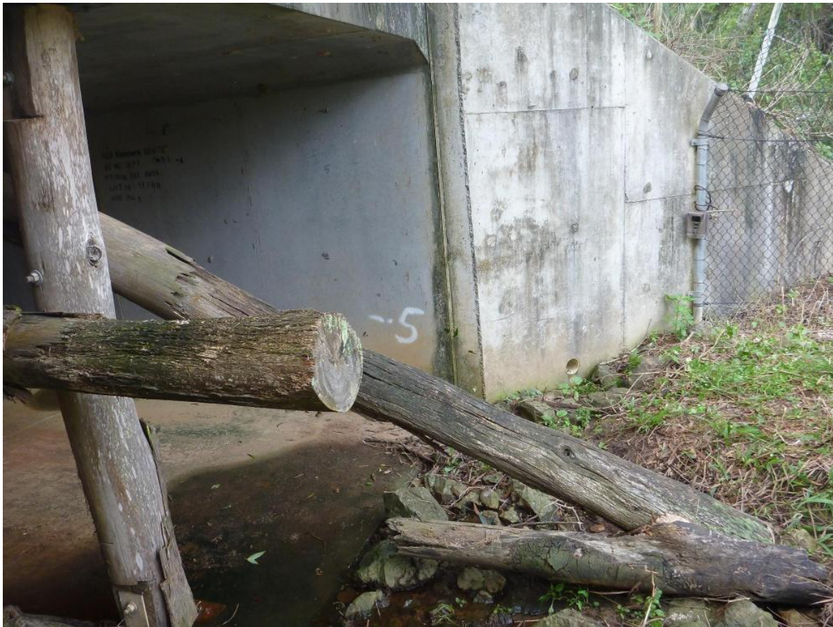
Termination of the fauna fence at the edge of the box culvert at Site 1. Short-eared Possums were recorded climbing over the fence and onto the top of the culvert.
